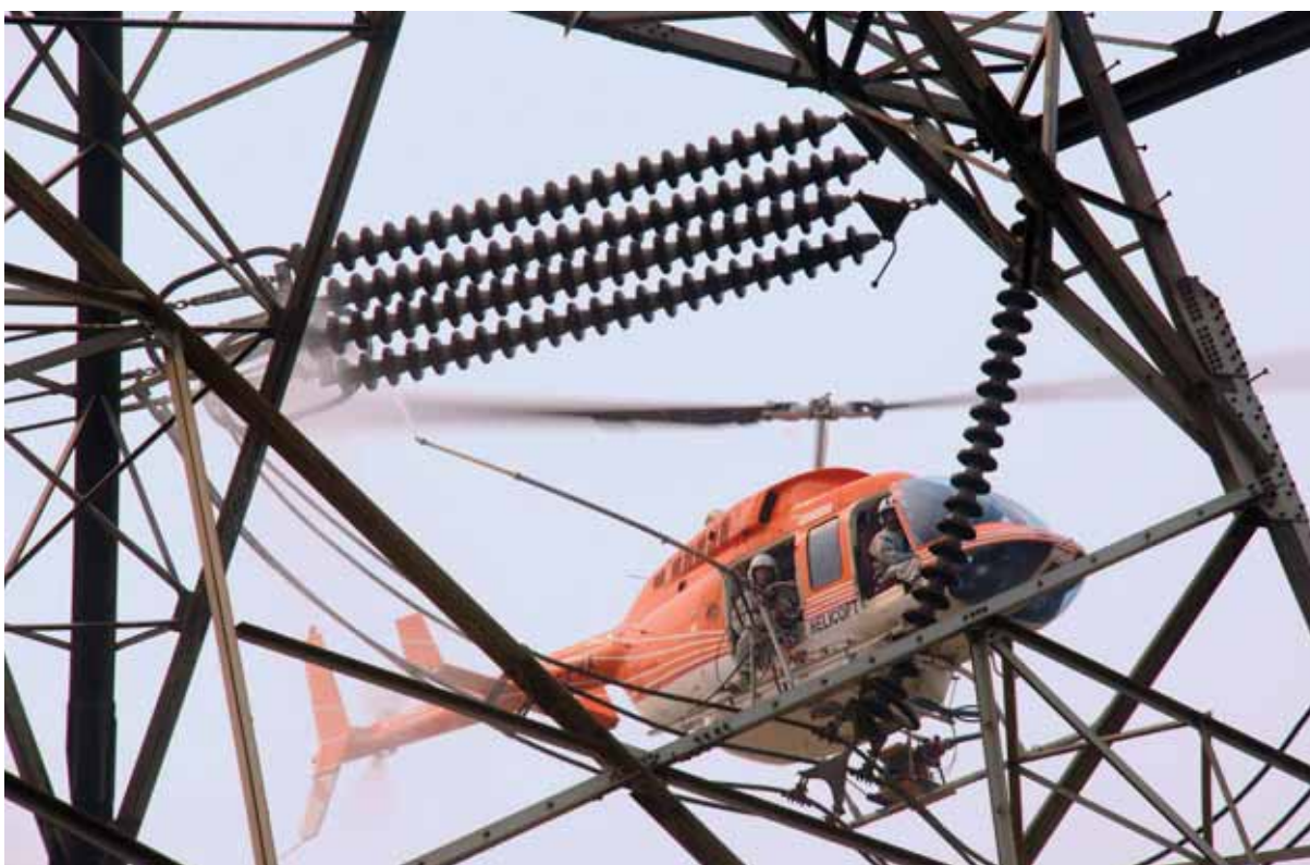
Bell 206L4 Helicopter doing hotline washing for transmission lines of Power Grid
